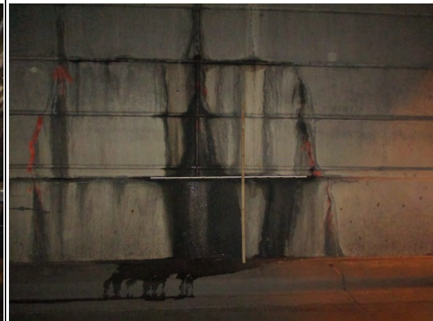
Condition State 4 Active dripping leakage
