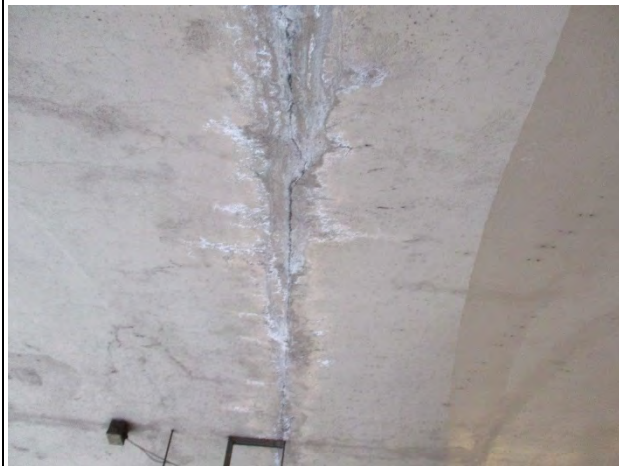
Condition State 2 Efflorescence at a construction joint in the liner
