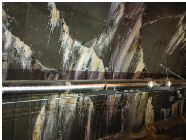
Condition State 3 Cracking with heavy efflorescence
