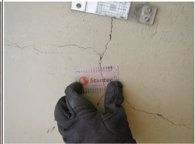
Condition State 3 Cracking in the tunnel liner above the springline
